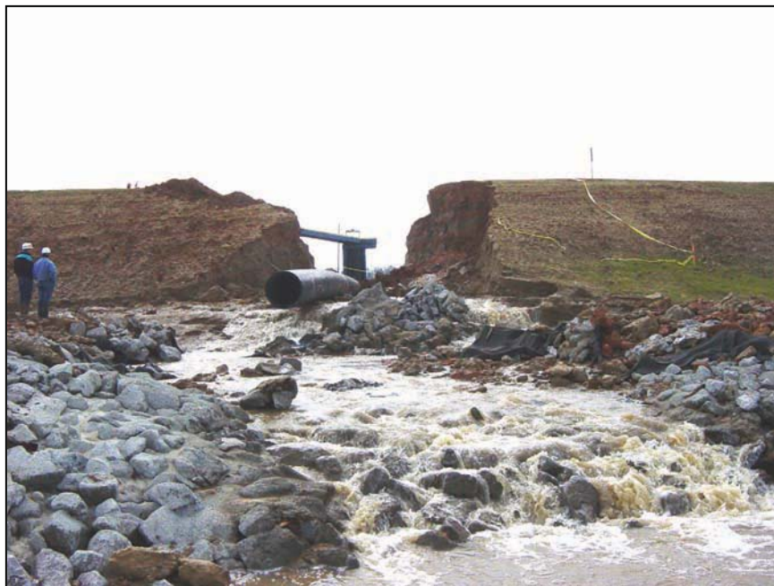
Figure B-8. —Looking upstream through the breach. Embankment was 18 feet high at breach.
